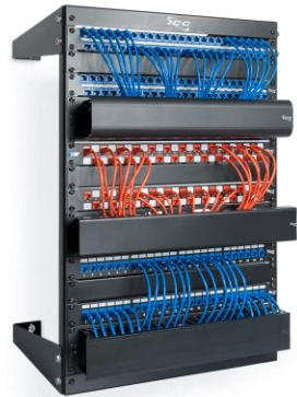
MDF Main Distribution Frame
